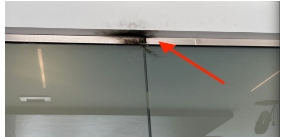
Smart Tint® electrical damage due to improper trim. (Non-conductive trims only)
