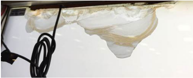
Smart Tint® electrical connections not sealed properly.
